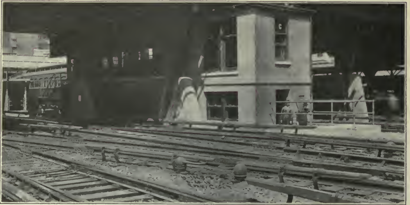
FIG. 508. THIRD RAIL CONTACT SYSTEMS. Construction at Switches, 600-Volt Under Running Third Rail Installation, New York Central & Hudson River Railroad, New York City.
